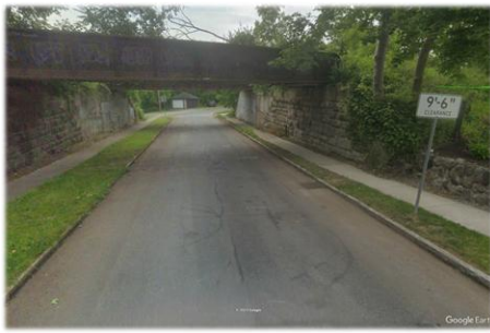
Greig Ter. Trestle clearance: 9'-6" west bound (one way street).
